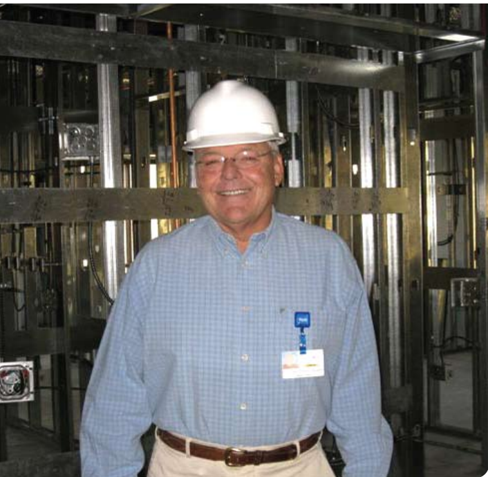
Dr. Thomas Broderick tours the Women's Imaging Center. Construction began in March and is scheduled to be completed August 3.
